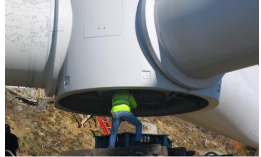
A technician inspects the hub before the rotor assembly is hoisted into place.
